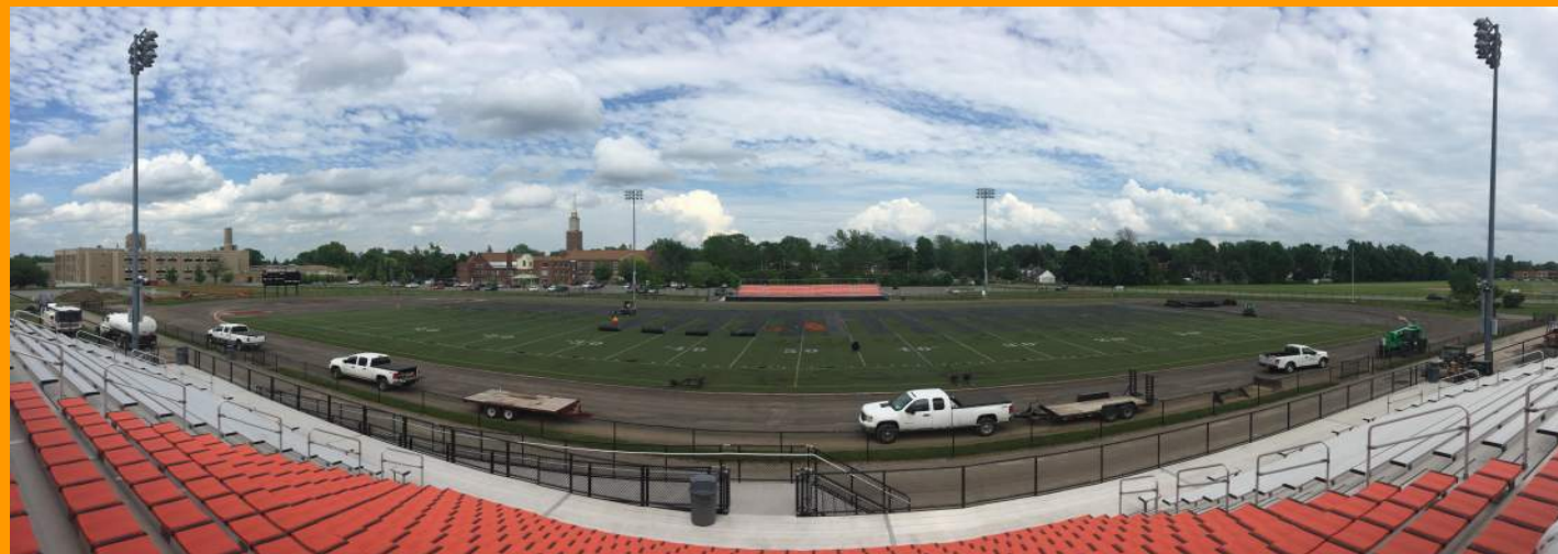
Removal of Original Turf Field and Shock Pad - Original Track Fully Removed
