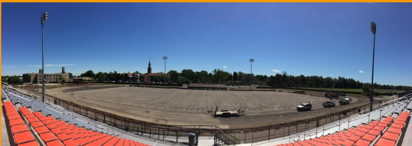
Original Turf Field and Shock Pad Fully Removed - Installation of New Stone Dust
